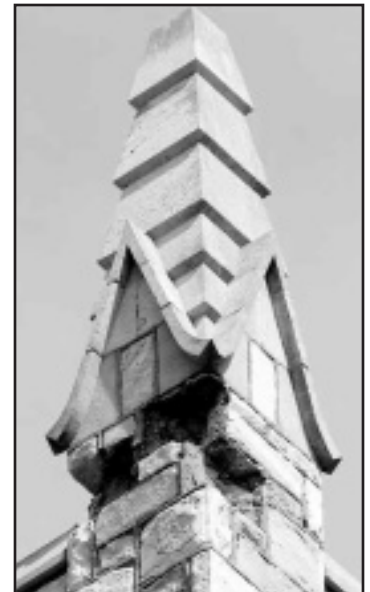
The Aug. 23 earthquake damaged this finial atop the church's steeple.
